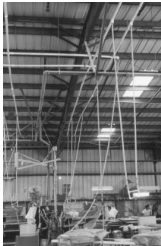
Figure 5-34 Overhead High- and Low-Pressure Vacuum Lines at Corsair Marine Facility [author photo]
