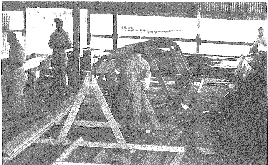
Fig. 2: The prefabricated frames for the 9.35 m canoe are erected on the building-jig.
