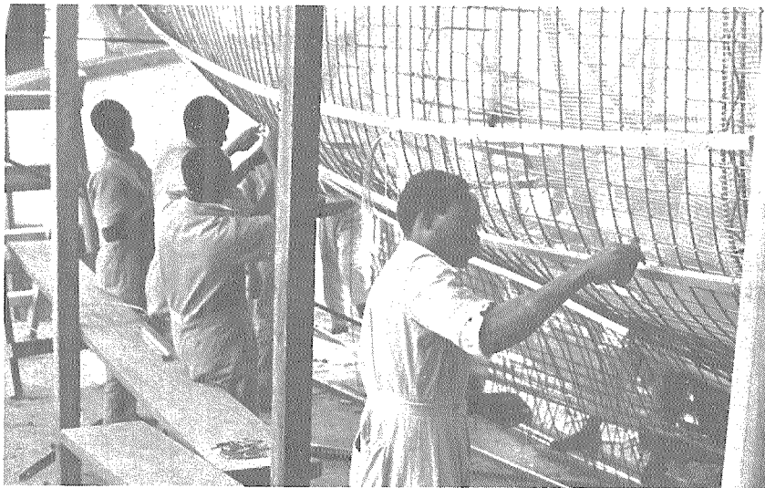
Fig. 10: Steel rods are tied longi- tudinally and transversely before the last four layers of mesh are applied.
